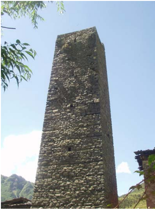
Laha Tower, repaired in 2006. It is one of several stone towers, some more than 30 meters tall, that still survive in Minyak.
