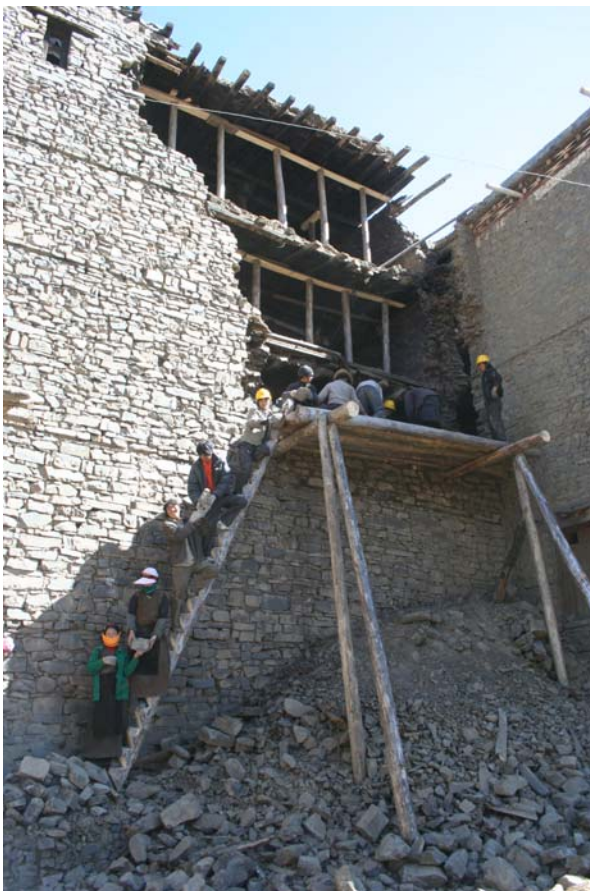
Top: Gongtsa House front façade. Bottom: repairs to south wall of Gongtsa House (October, 2006). Temporary shoring is visible where the wall has been dismantled.
