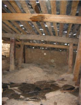
Inadequate coverage of slate results in water infiltration soaking the roof frame and the fabric beneath it. This leak showed repercussion through the building down to the ground floor.
