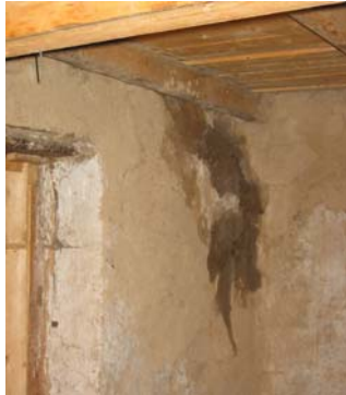
Moisture infiltration at the SE corner of the upper floor of the new portico
