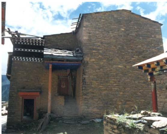
Exterior north wall of Protector Temple, with clear separation between earlier structure and new portico.
