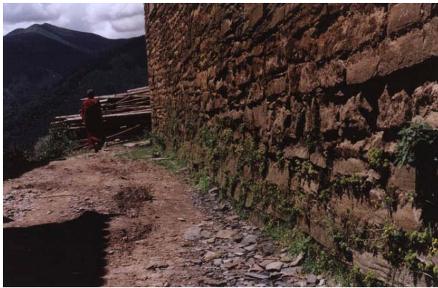
South exterior wall of the Protector Temple with extensive plant growth at the base, evidence of excess moisture in the building fabric. The roof of the nearby kitchen (note shadow) and the roof of the Protector Temple shed large amounts of water into this narrow alley during downpours. Lack of adequate drainage results in moisture creeping up the walls of the building through capillary rise.
