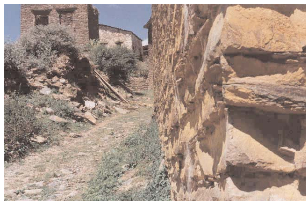
Protector Temple / Exterior West Wall View of base of wall looking north, note plant growth at base of wall August, 2002
